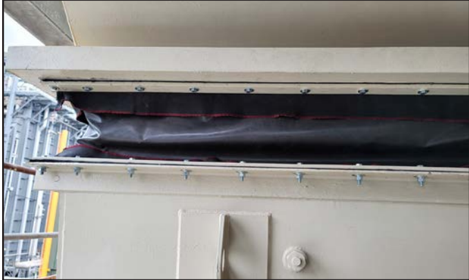
A new composite fabric expansion joint is installed with PTFE flange gaskets, new hardware assemblies, and the previously removed backing bars
