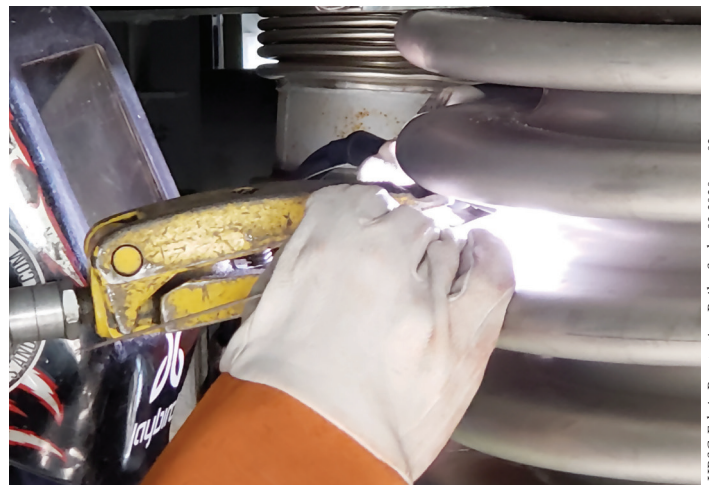
HRSG-Fabric Penetration Boiler Seals_05.2020_rev02
