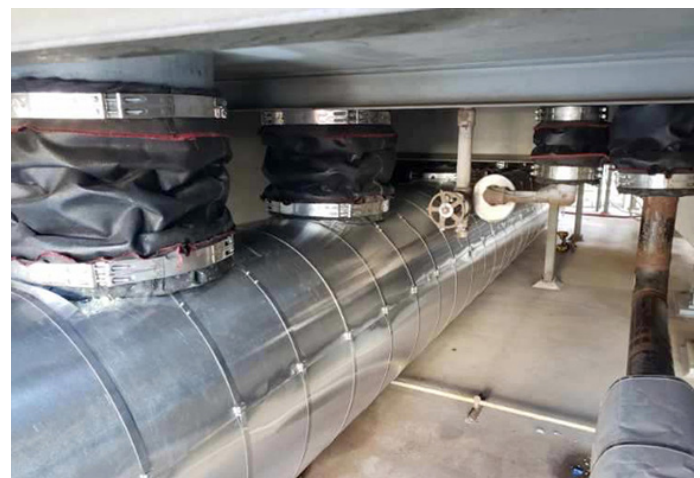
Fabric penetration seals (bottom of HRSG) installed compressed in the cold position, before insulation complete
