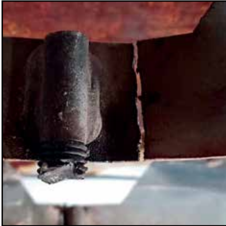
Typical scallop bar crack
