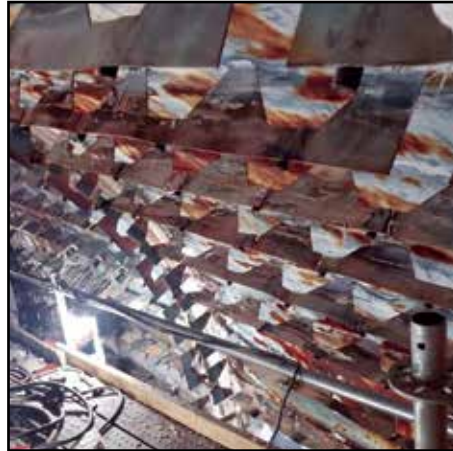
Scallop bar distortion and cracks
